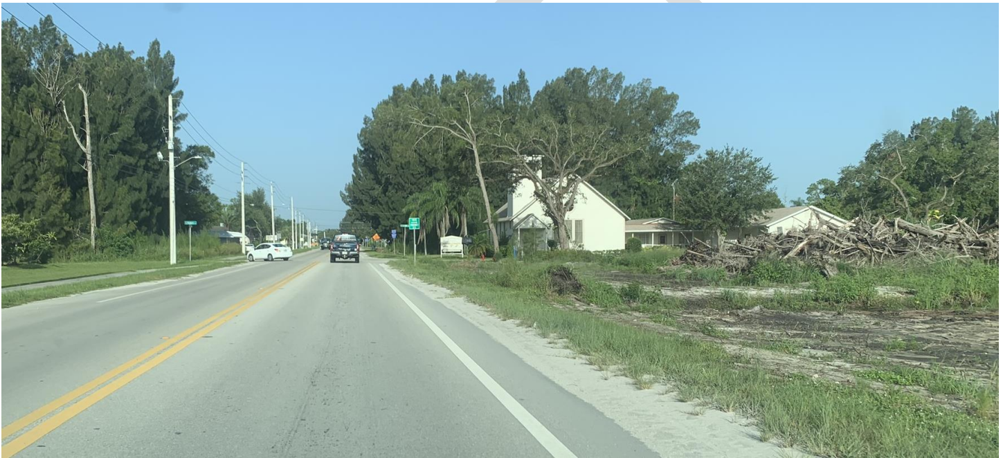
Figure 5 – Sand and grass encroaching on bike lane, westbound on CR 512 (west of I-95)
